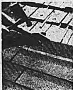
Many Title I loans are used for reroofing. Here, heavy-weight asphalt shingles are being applied directly on old roof surface, a procedure more inexpensive than removing the old material first. The average Title I roofing loan is for more than $700.
